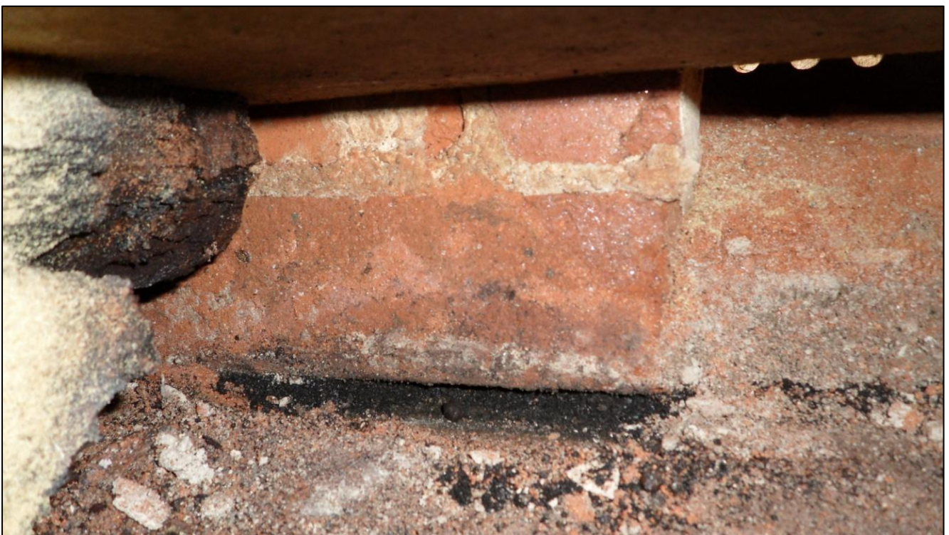
Photograph 2 - Back room of the Building on the Post Office side showing water droplets on the bearer:
