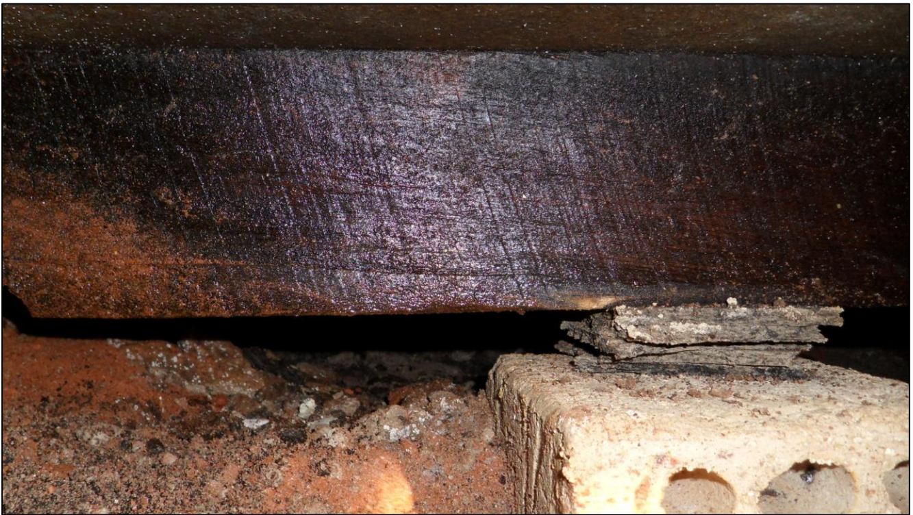
Photograph 1 - Back room of the Building on the Post Office Side showing damp on the bearer:
